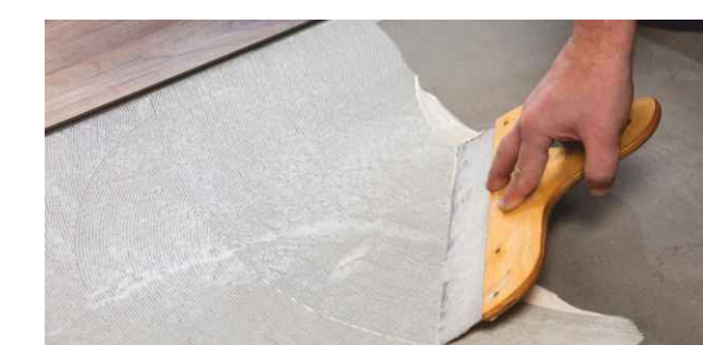
Cracking at corner & around cuts may be caused by improper conditioning, improper bonding, poor planning, avoid all these to prevent cracking at corners.
