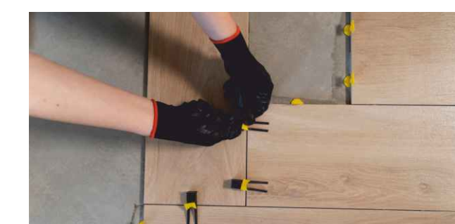
Extra care required in vertical pasting of Laminated sheet there is possibility of bubbles due to lack of uniform pressure
